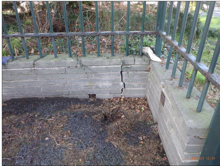
Figure 5 - Damage to retaining wall
