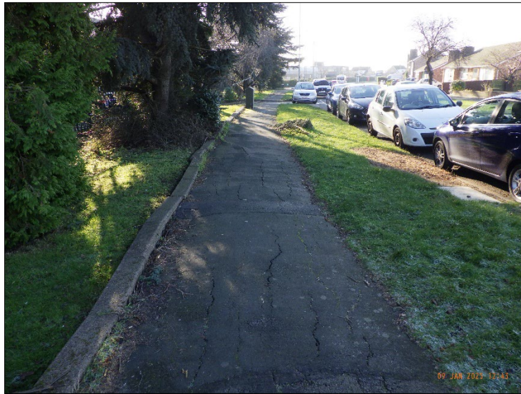
Figure 1 - Damage to footpath
