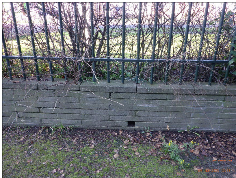
Figure 6 - Damage to retaining wall
