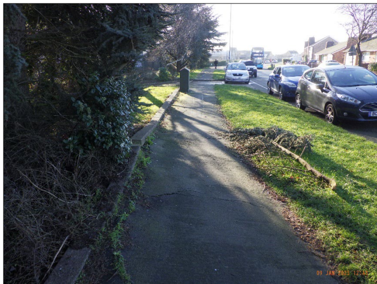
Figure 2 - Damage to footpath
